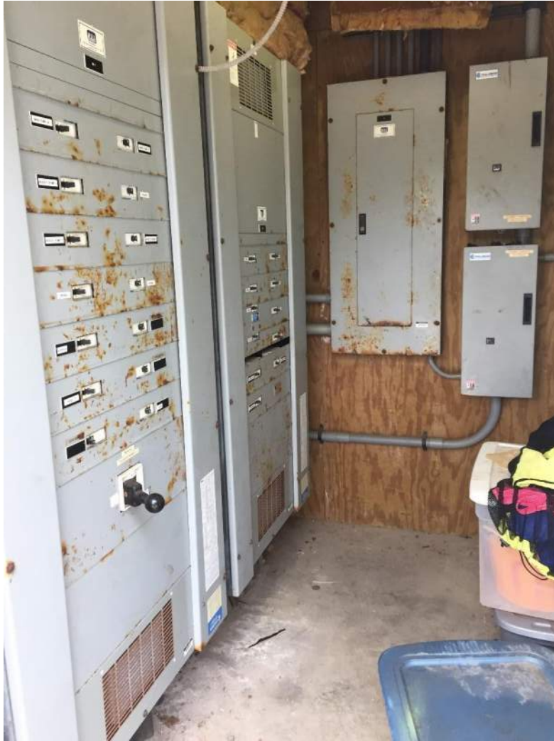
Electrical Control Room (note corrosion)
