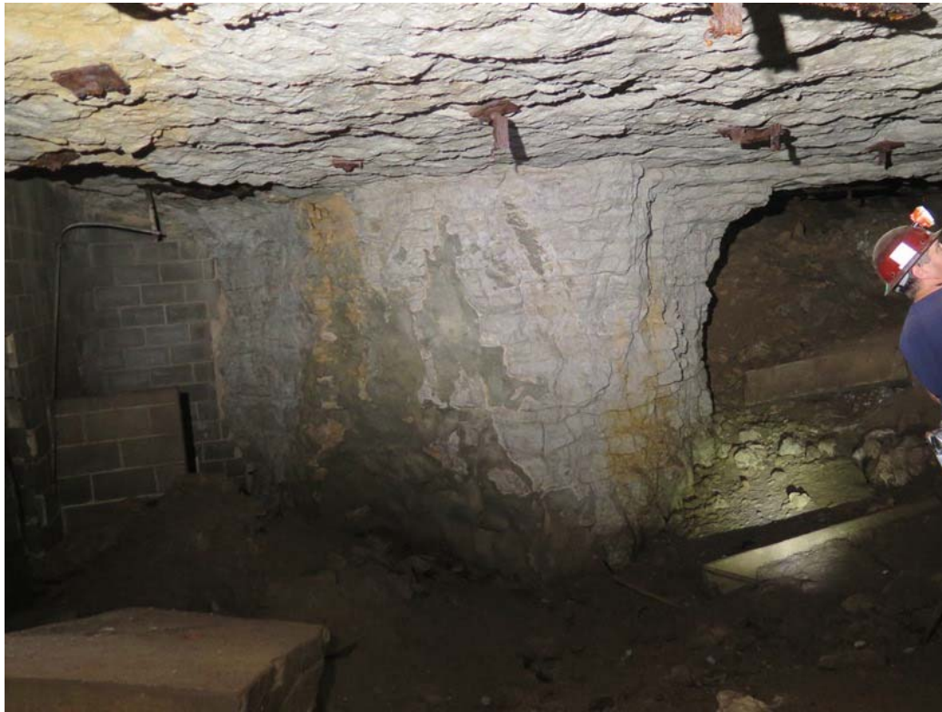
Photo 27: Looking southwest at Pillar 4, masonry along Portal 2 on left, Portal 1 on right. Guniting and staining on pillar may indicate a mud seam.
