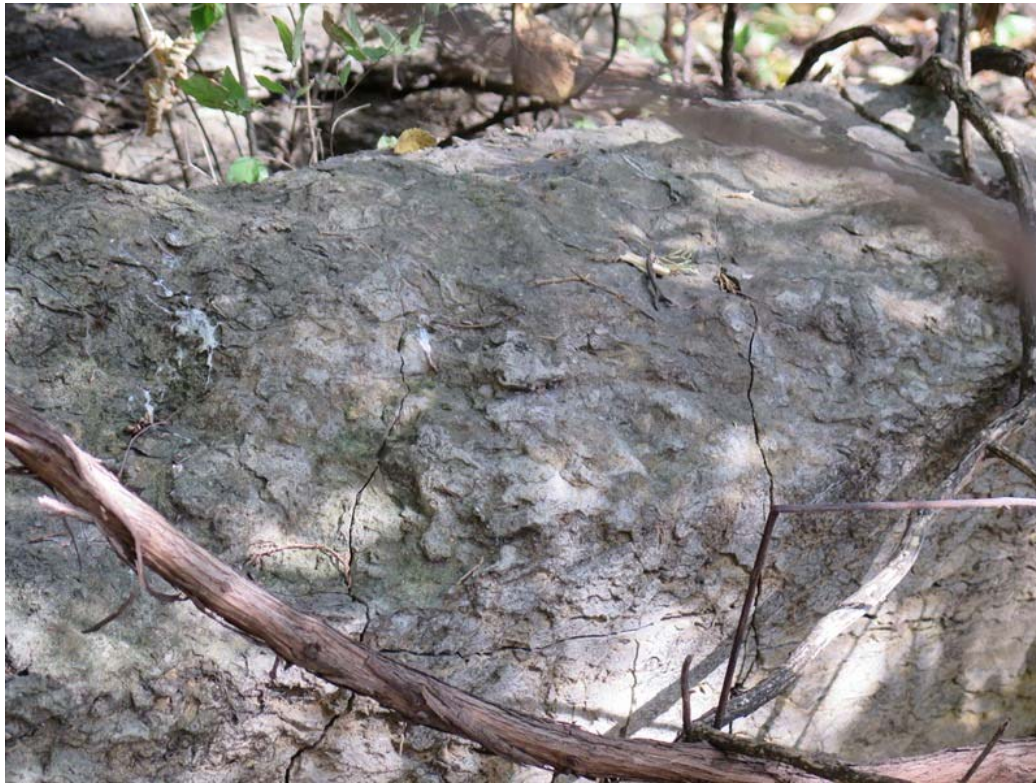
Photo 11: Frost fracturing of rock near top of highwall above Pillar 4.
