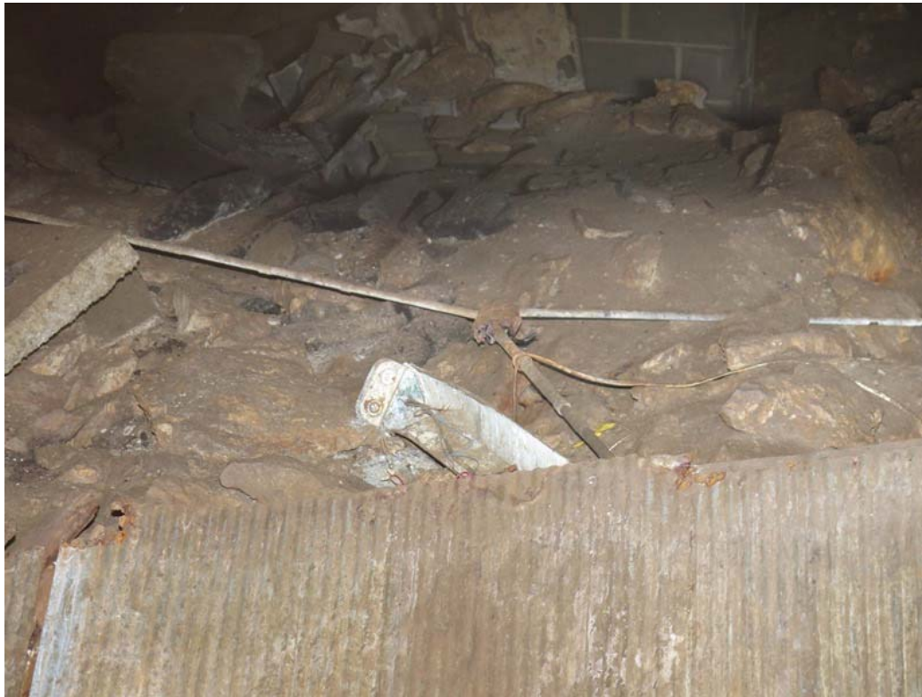
Photo 21: Looking north into Portal 2. Corrugated metal at bottom formerly blocked the portal. Fill material, piping, and light fixtures visible on floor.
