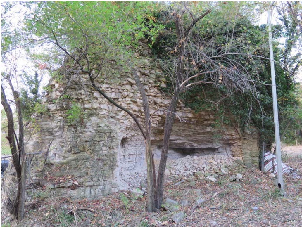
Photo 6: Looking southwest at undercut on north side of Pillar 14.
