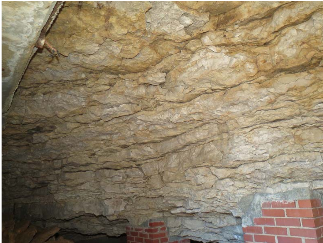
Photo 20: Looking west-northwest into Portal 2, loose strata in ledges.
