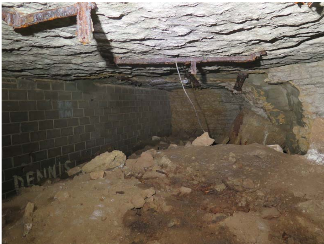
Photo 26: Looking north between masonry wall inside Portal 1 on left and Pillar 1 on right. Heavy gunite and staining visible on Pillar 1.
