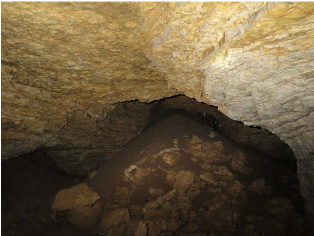
Photo 54: Looking south at, from left to right, dome-out, Pillar 12, dome-out material and Portal 5 fill, and Pillar 10. Dome is highly developed in this area, and may indicate a risk of a dome-out.
