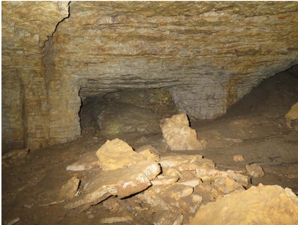
Photo 51: Looking east, rockfalls in foreground. From left to right in background are Pillar 16, dome-out, Pillar 11, and dome-out.
