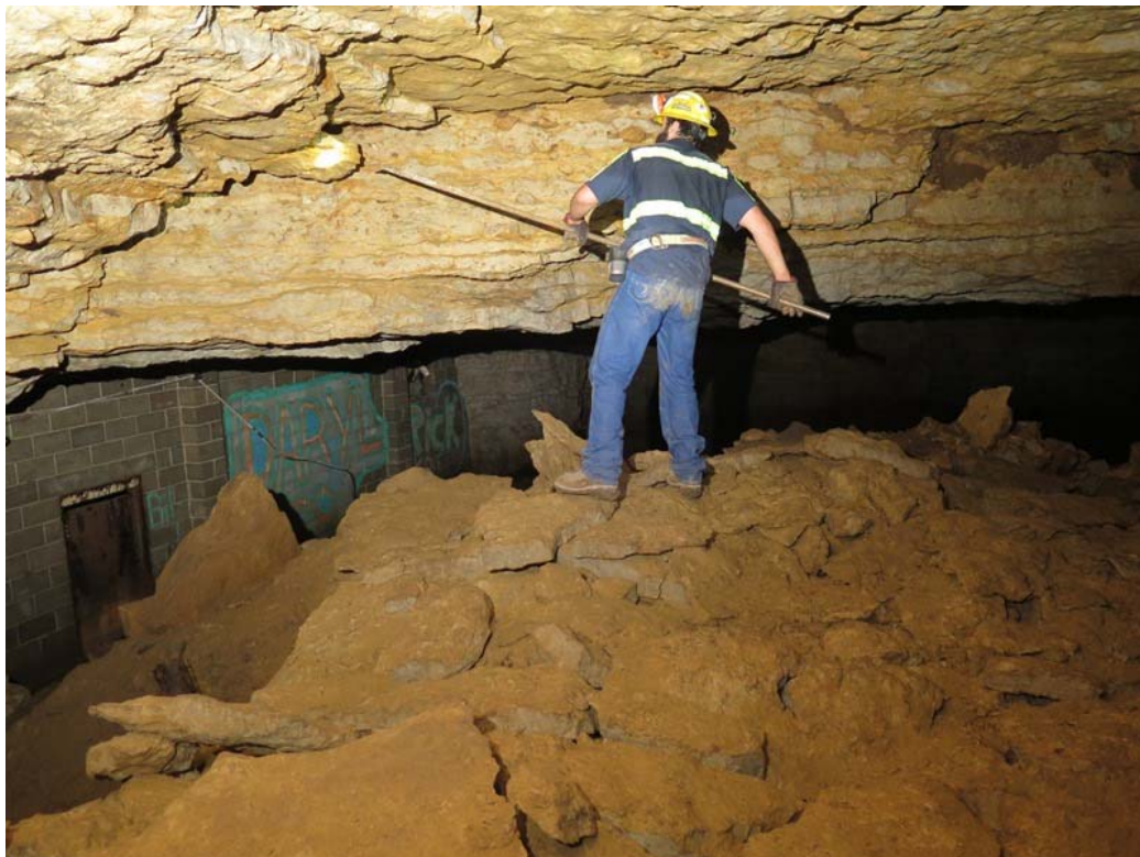
Photo 42: Looking northwest at scaling in dome north of Portal 4. Note original level of mine roof. Graffiti on masonry wall was dated 1968. Door on left is the east side of the door shown in Photo 40.
