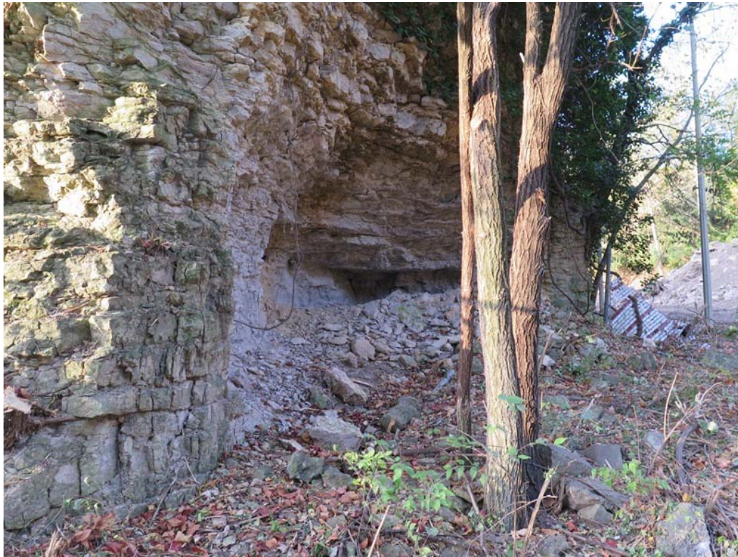
Photo 7: Looking west at north side of Pillar 14 showing undercut and overhand.
