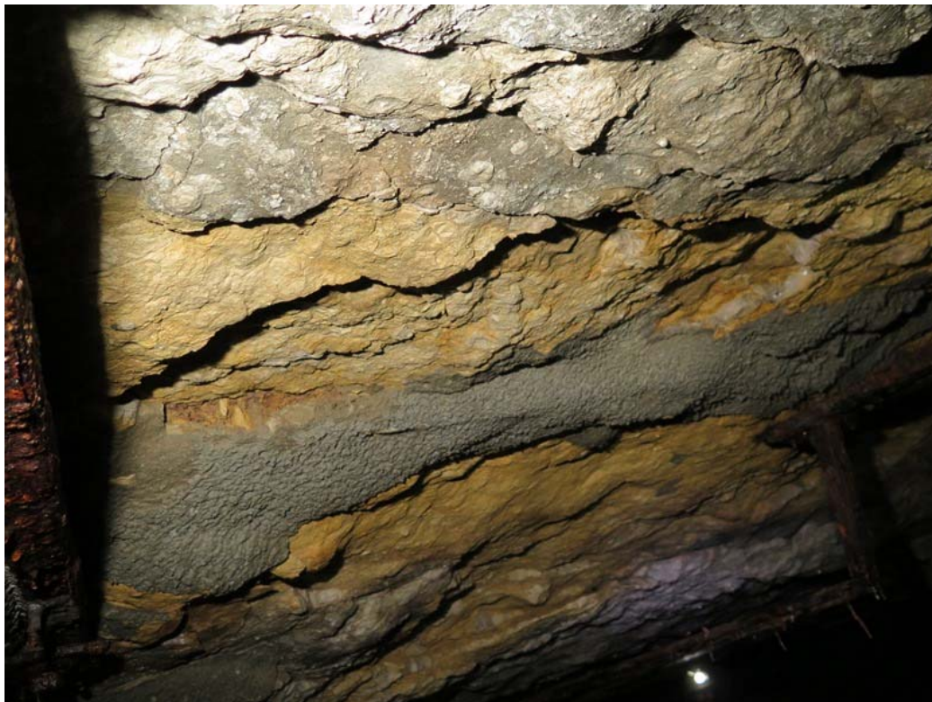
Photo 38: Mud seam with remnants of gunite in room north of Portal 3.
