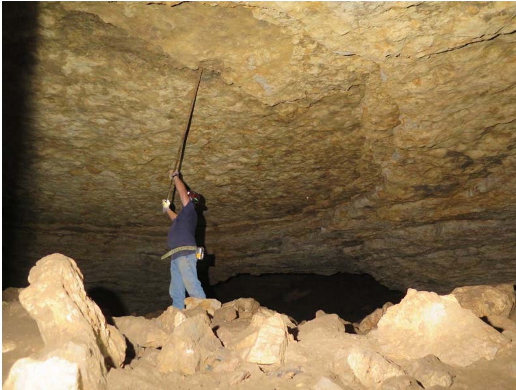
Photo 41: Looking east-northeast at scaling in dome north of Portal 4. Pillar 7 is shown on the left, Pillar 10 on the right.
