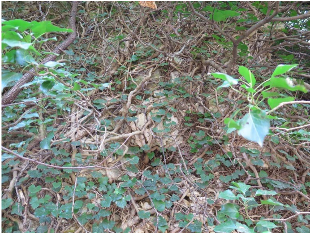
Photo 8: Ivy on northwest side of Portal 14. Note loose rock held in place by vines.
