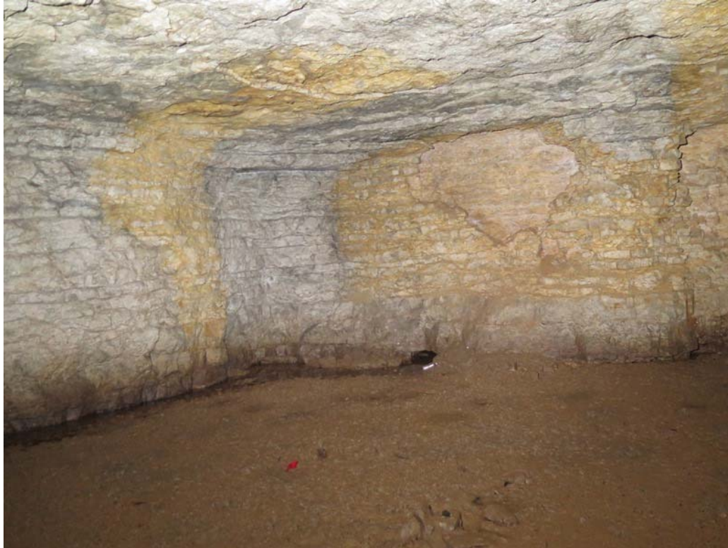
Photo 49: Looking northwest in room north of Portal 4 dome. Floor is mud-covered and has historically been inundated. Dark feature near lower center of photo is a source of ongoing inflows.
