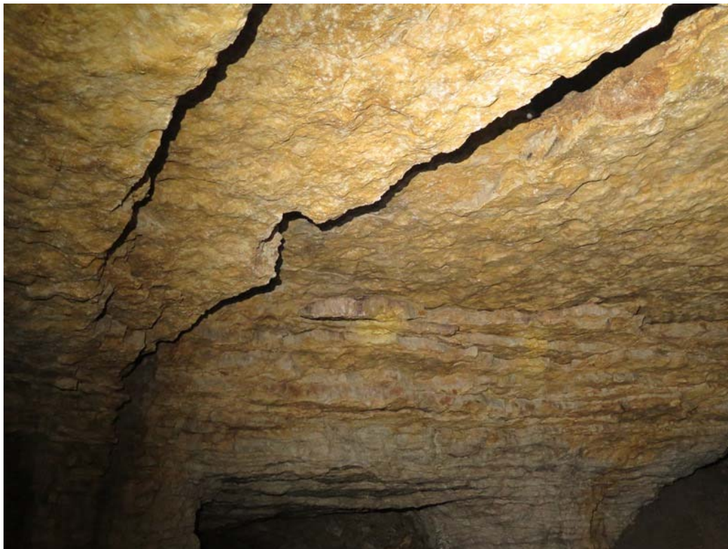
Photo 52: Looking southeast along mud seams, showing locations of rockfalls. Pillar 16 is on the left, Pillar 11 on the right.
