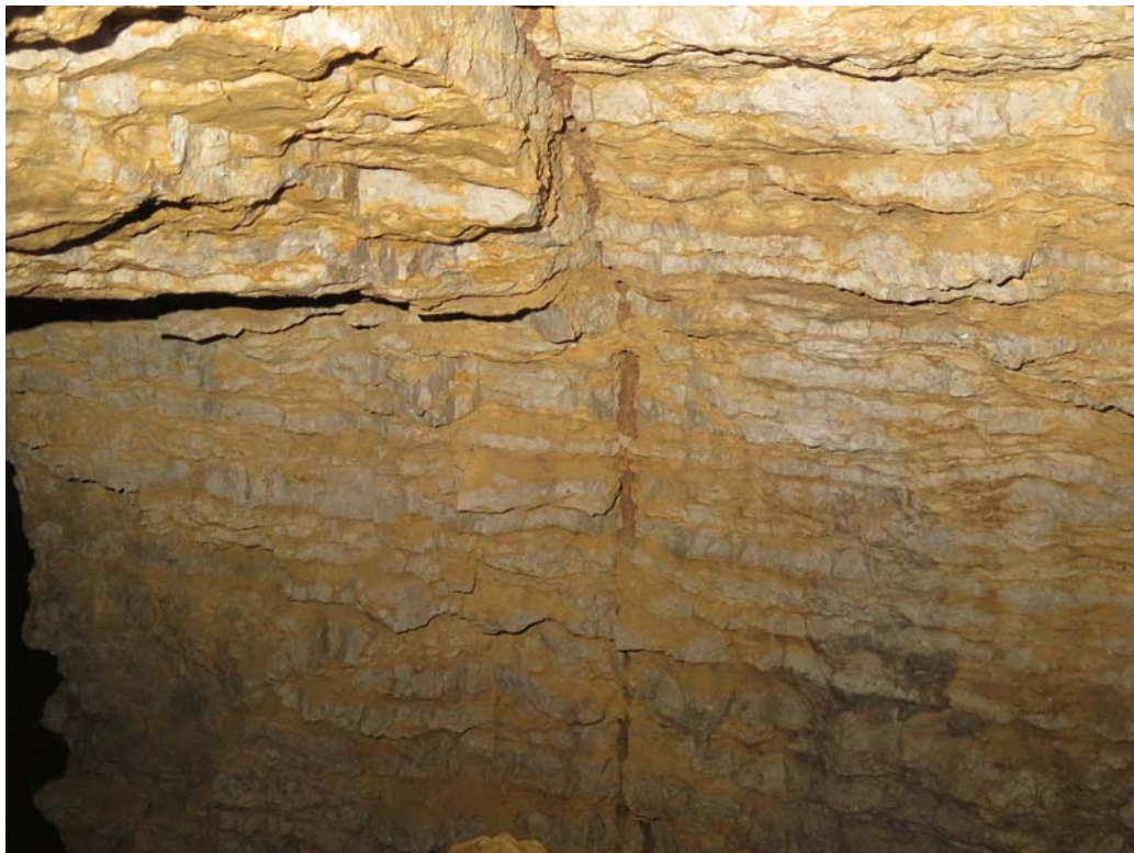
Photo 48: Looking northeast at continuation of mud seam visible in Pillar 7.
