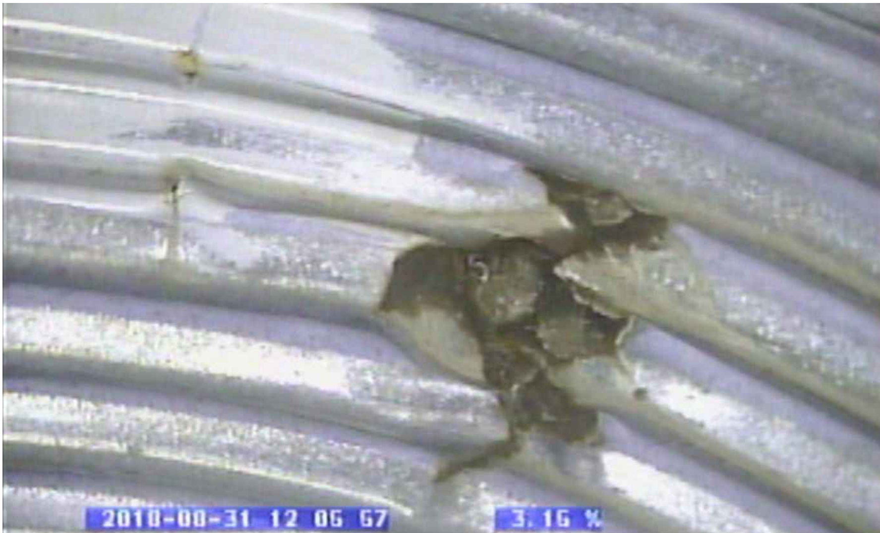
POINT REPAIR STA: 1+62.50
