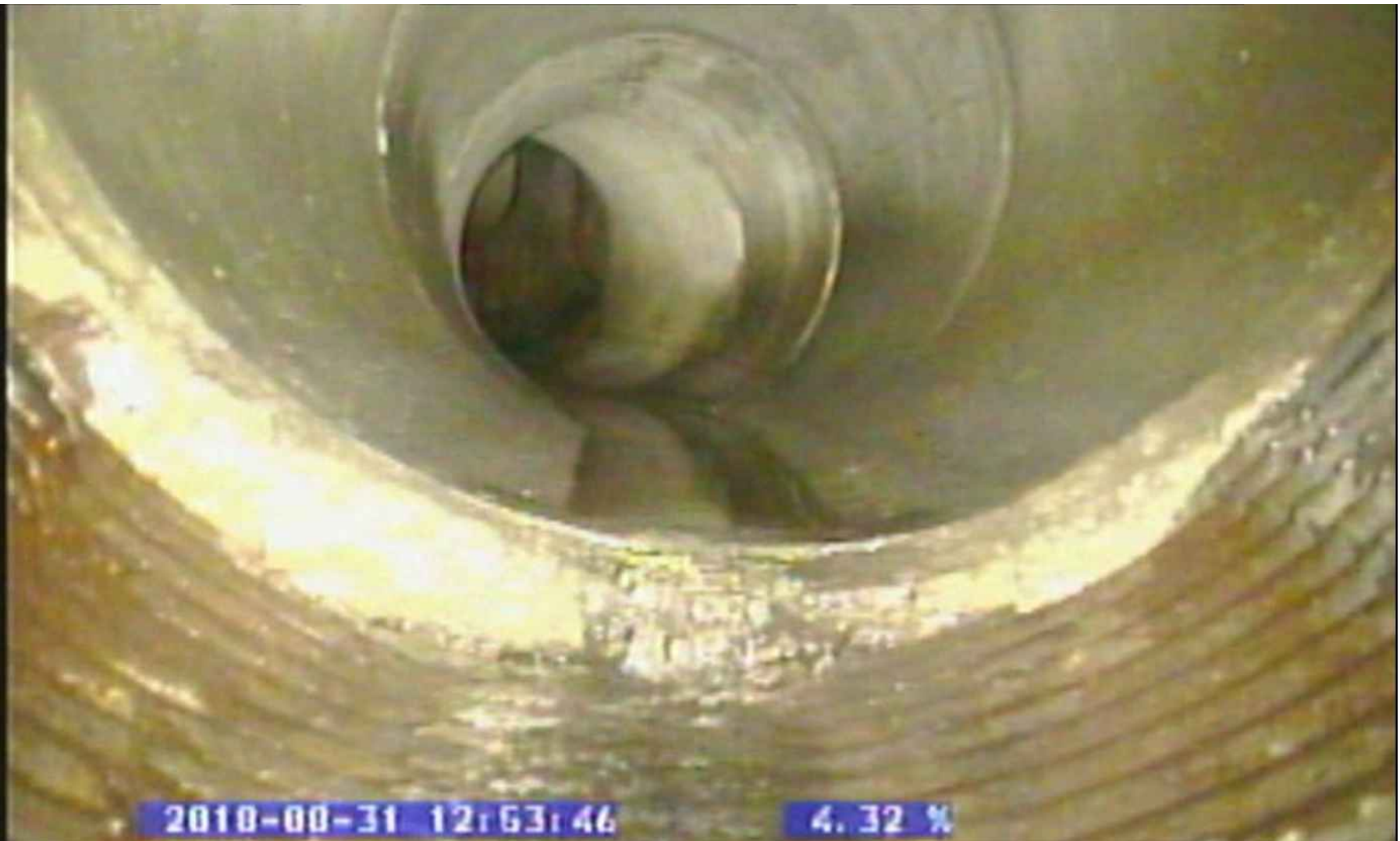
POINT REPAIR STA: 7+44.27
