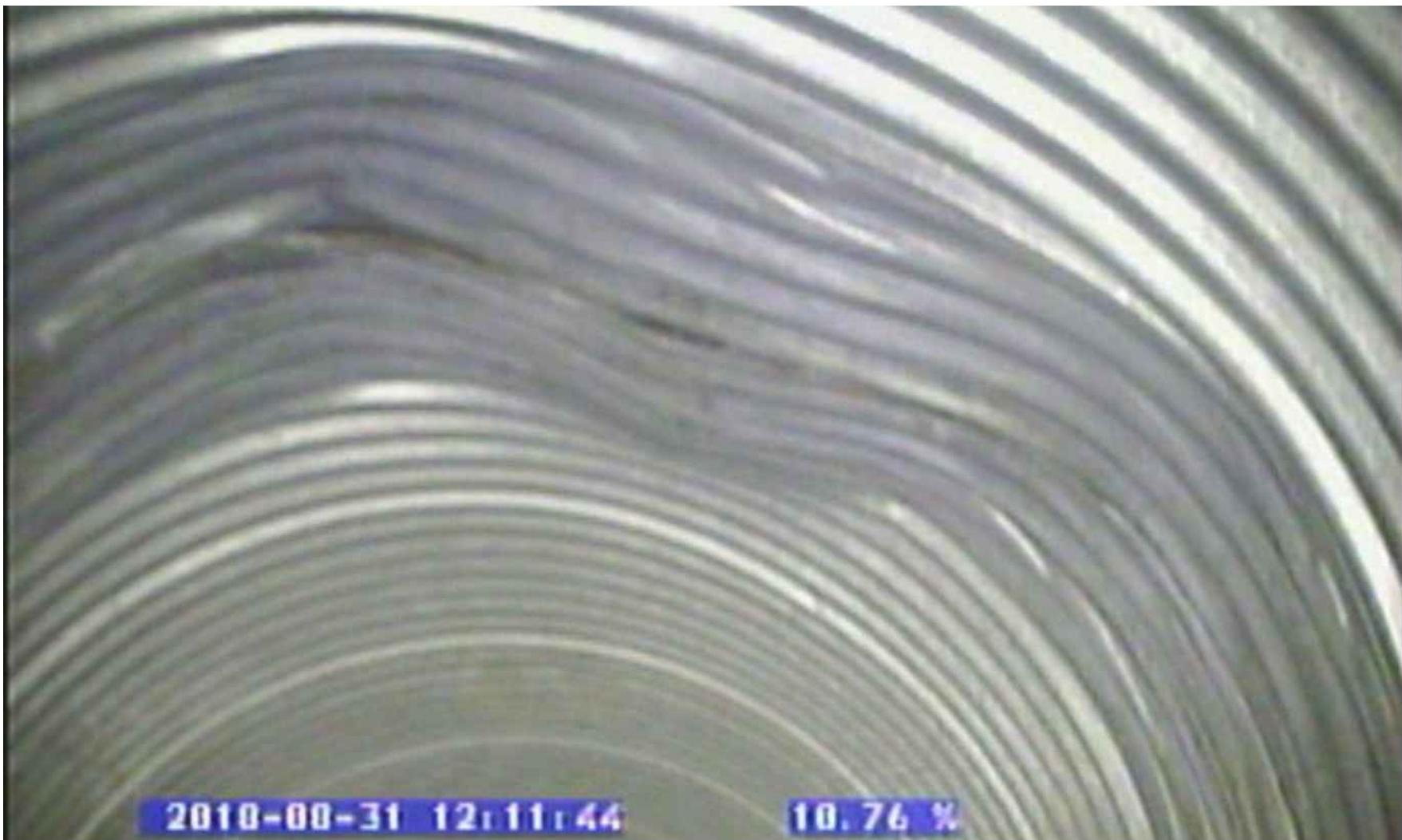
POINT REPAIR STA: 2+44.40
