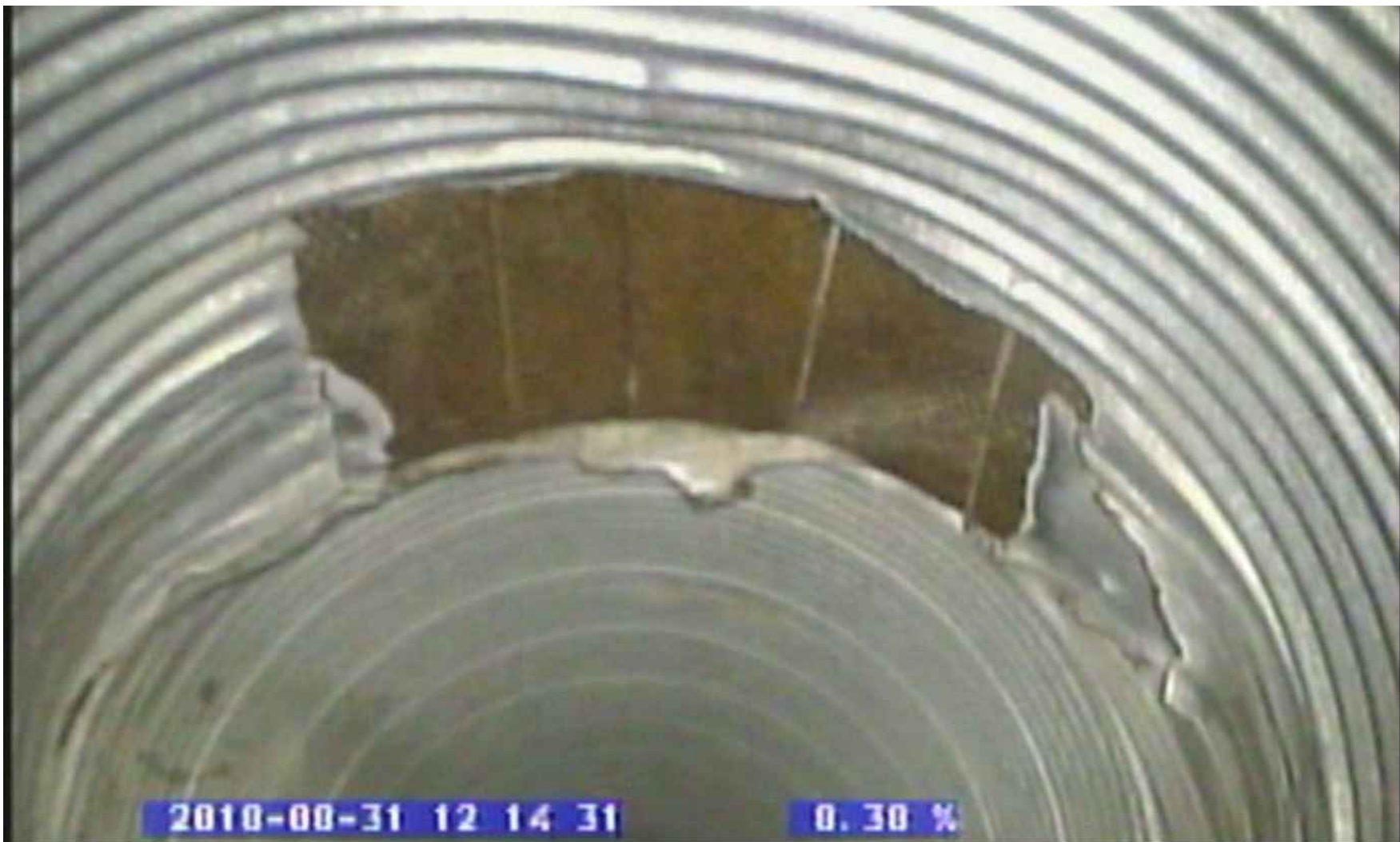
POINT REPAIR STA: 2+65.20
