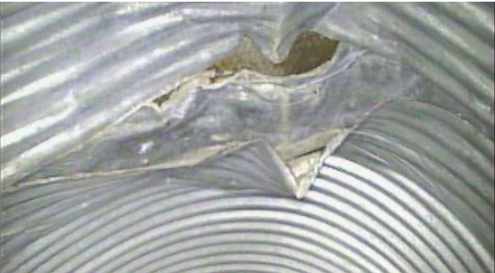
POINT REPAIR STA:1+73.20
