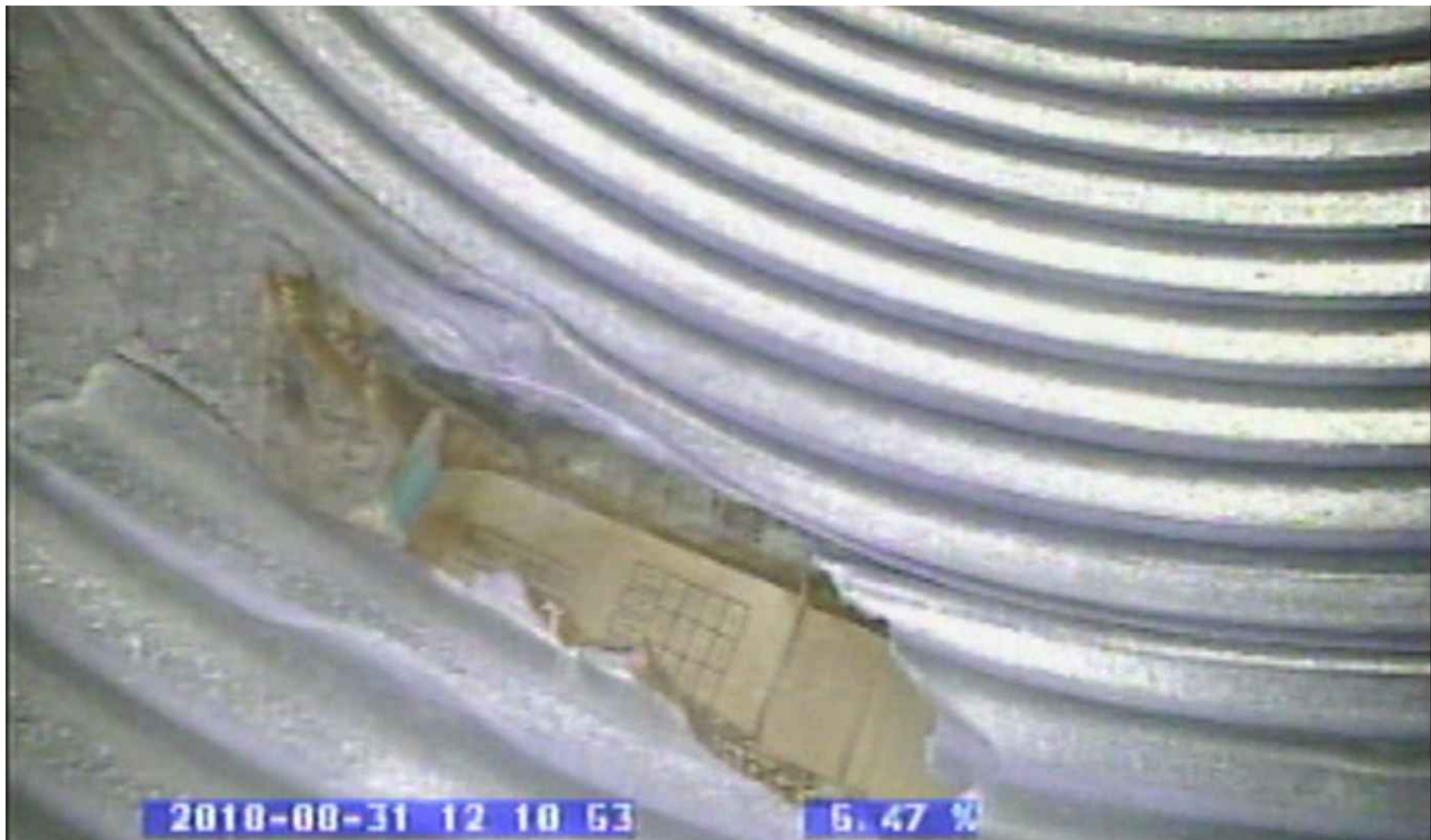
POINT REPAIR STA: 2+35.50
