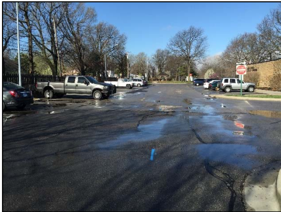
Ponded water in lot southeast of Community Center
