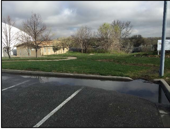
Ponded water at flume in lot north of Community Center
