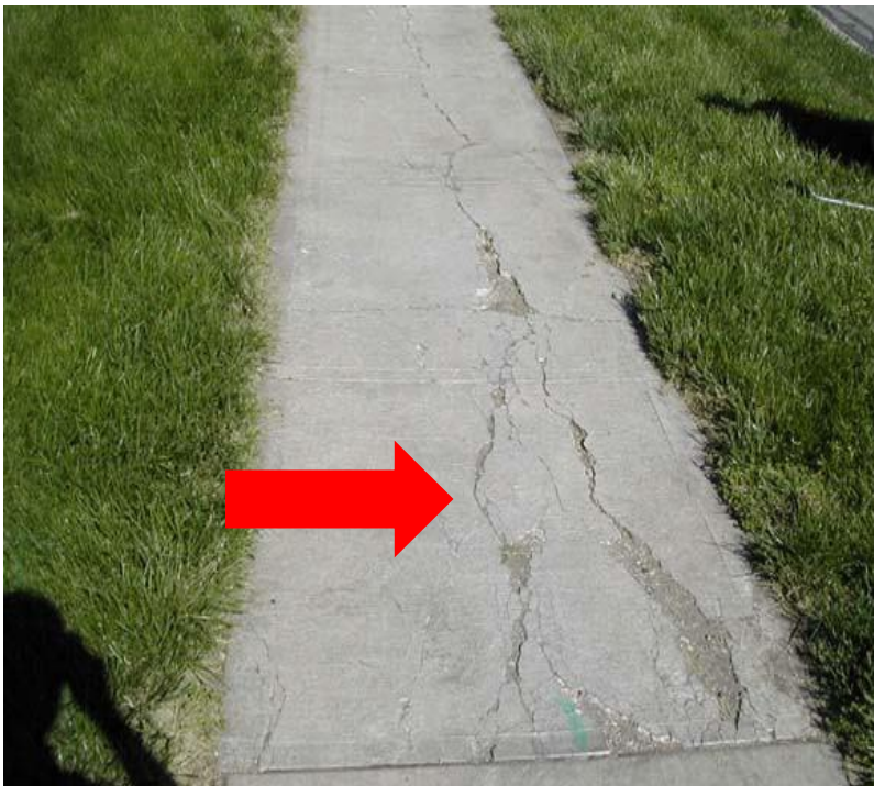
Figure 2H – High Severity “D” Cracking
