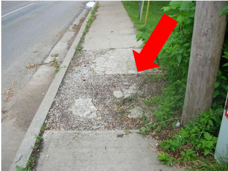
Figure 11H – High Severity Surface Defects
