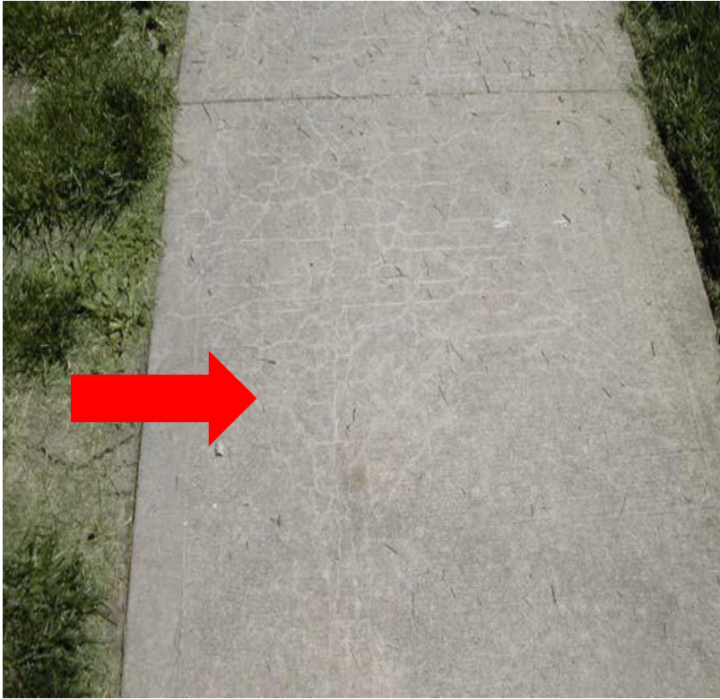
Figure 2M – Medium Severity “D” Cracking
