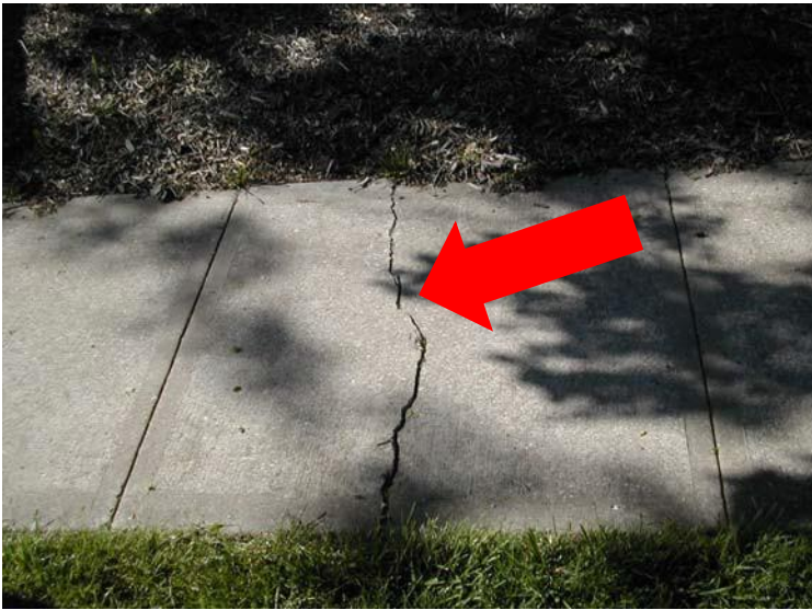
Figure 5L – Low Severity Linear Crack
