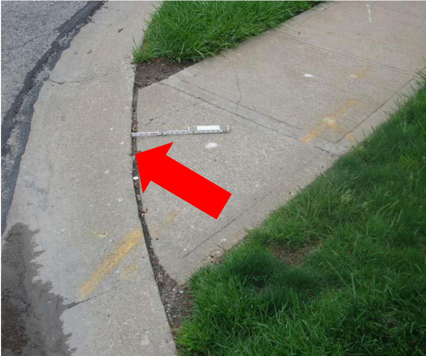
Figure 4L – Low Severity Gap
