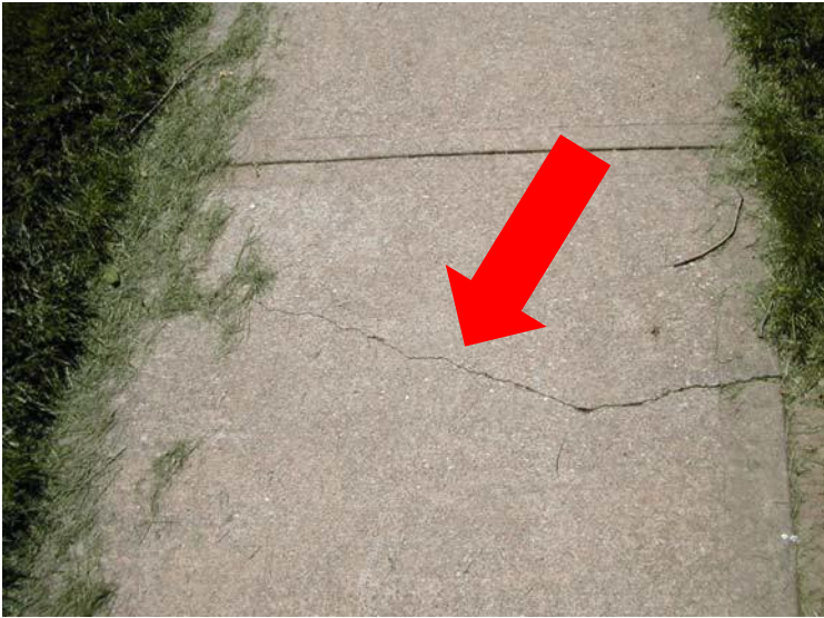
Figure 5N – Non-faulted Linear Crack
