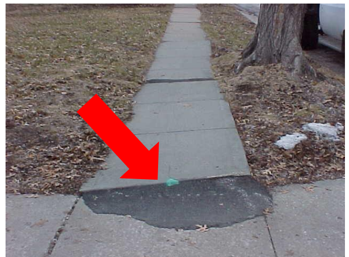
Figure 3P – Patched Fault
