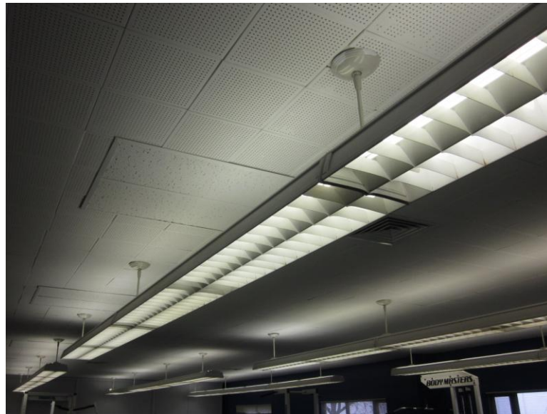
Figure 4.10.A: Typical Rental Room Lighting
