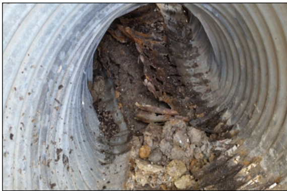
Condition of Existing Pipe showing rust
