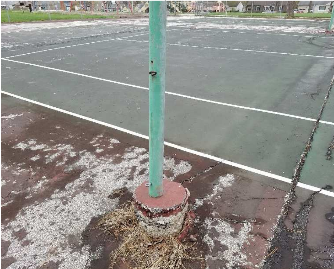
Picture 4- Settled pavement around net post
