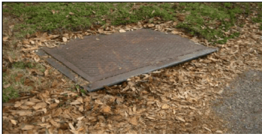
Clogged catch basins cause street flooding
