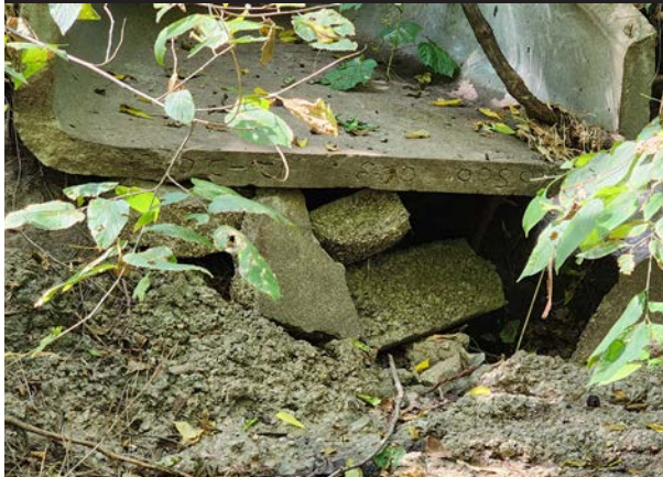
Figure 14. Storm outfall damage detail, Reach 2
