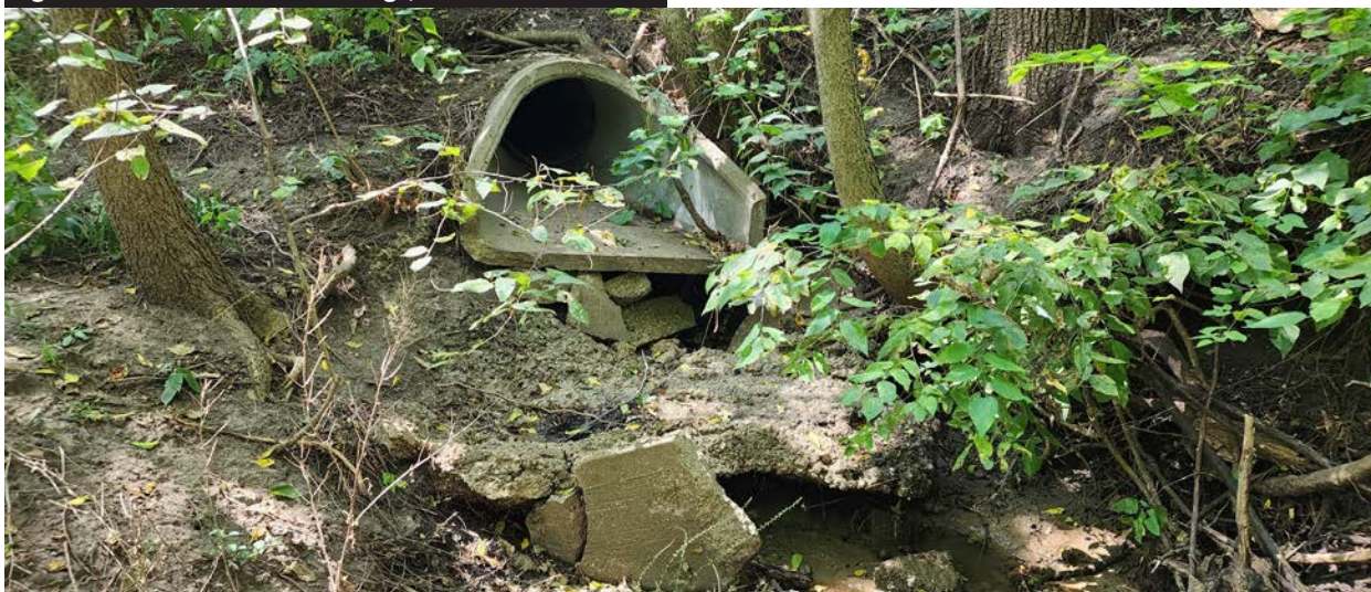
Figure 13. Stormwater outfall damage, Reach 2
