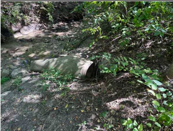
Figure 17. Stormwater structure erosion, Reach 3
