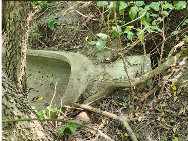
Figure 18. Stormwater structure erosion, Reach 3
